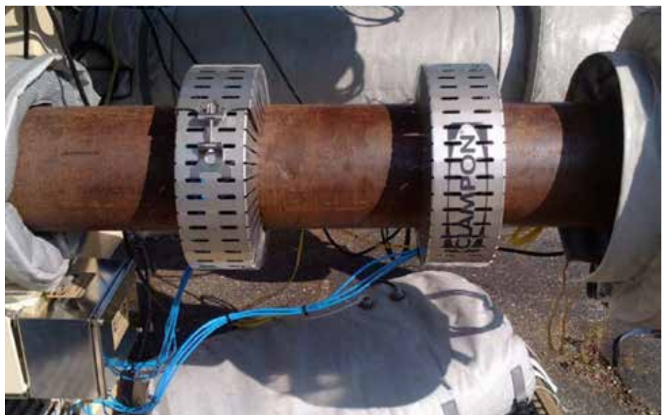
Figure 6. Topside CEM being installed for field testing on a 6 in. pipe. Transducers under protection covers, to be covered by insulation.
