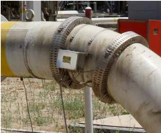
Figure 1. CEM on 24 in. gas pipeline, with ultrasound transducers under two circumferential protection covers. Signal paths set up to monitor generalised corrosion on top, bottom, and sides.
